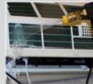
Clean coils from the front
