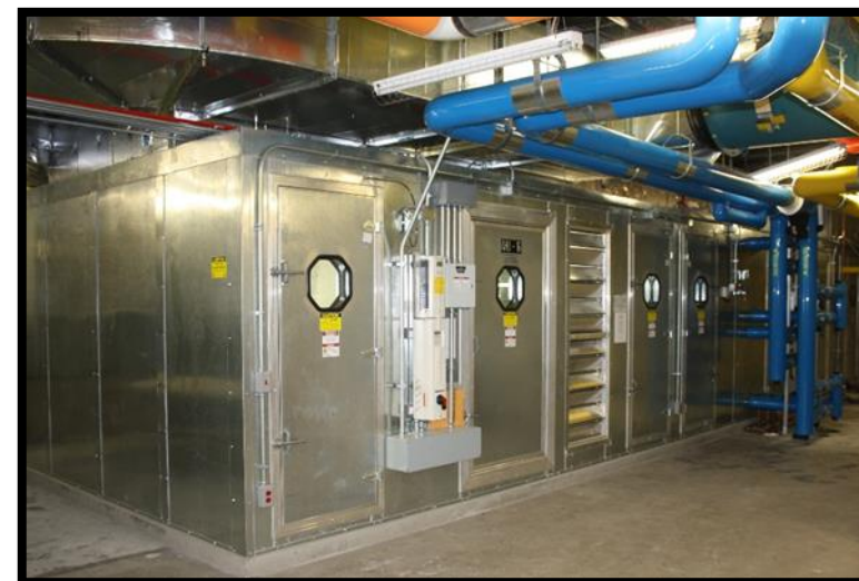
Built in place AHU
