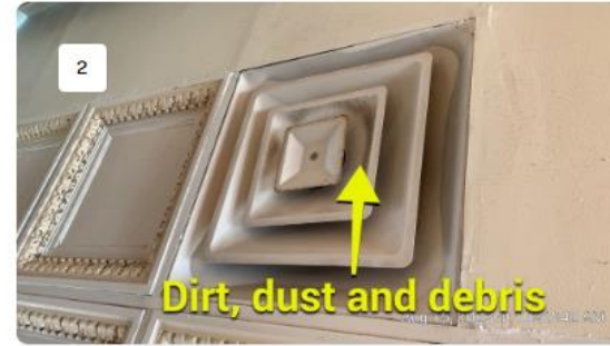
Ceiling supply vent
