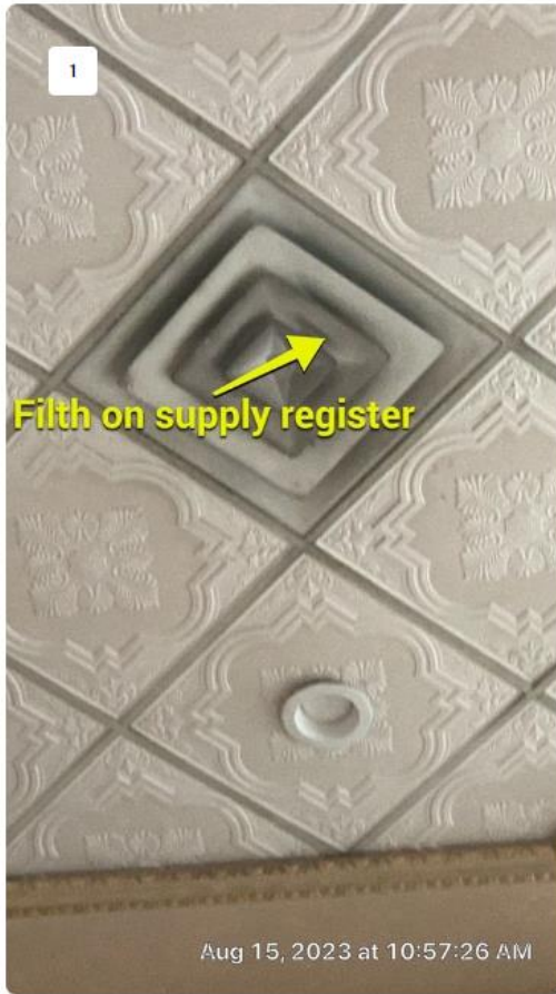
Ceiling supply vent
