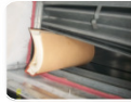
Soot can contaminate an HVAC system through many points of entry. When fire dampers are braced open. In the event of a fire, smoke and soot will be transferred throughout the HVAC system.
