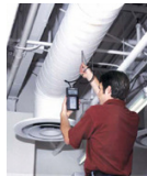
Image of duct traverse reading courtesy of www.achrnews.com
