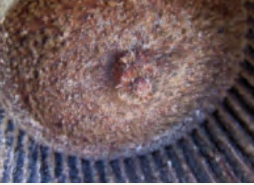
Dirty Fan: Blowers such as this can become heavily contaminated and require cleaning for maximum efficiency.
