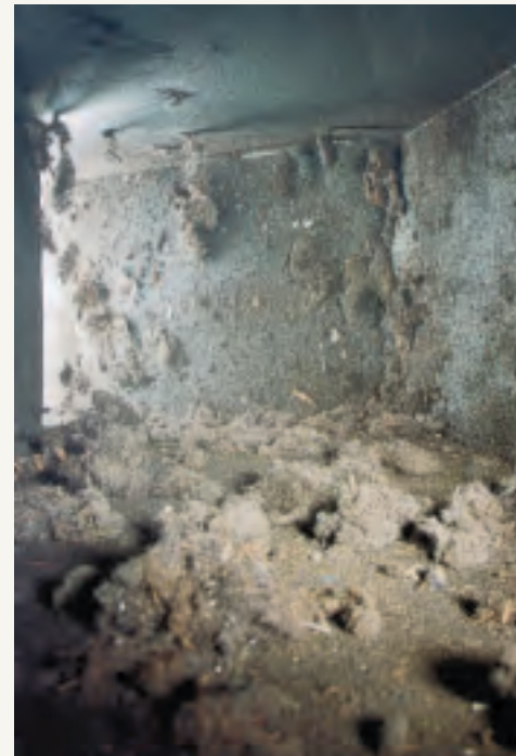
Dirty Duct: Accumulations of dust and debris within HVAC ductwork can contribute airborne particulate within a home or commercial building, while also reducing air flow and increasing energy consumption and related costs.
